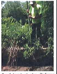
Canal Invert at pipe discharge beneath Norwood Road @ EL. 248.48 (survey shot taken during July 2013 survey)
