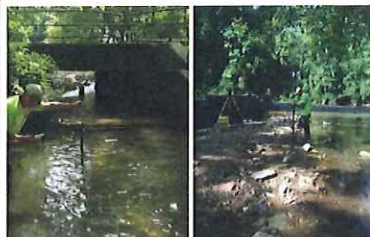
LEFT PHOTO: Point No. 1537 - Silt Accumulation @ EL. 250.63; RIGHT PHOTO: Point No. 1535 - Bottom of Scour @ EL. 247.73
