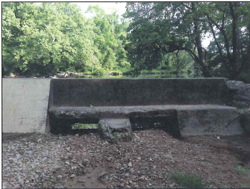
Photo 4 (06/24/14): Downstream End of Canal Intake (Looking Upstream) (Note Change in Silt Accumulation from 05/31/13)
